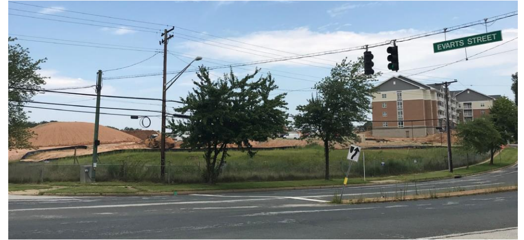
View of the Phase 3 site and Phase 2A under construction, looking northwest from Brightseat @ Evarts; RDA mass grading work underway
