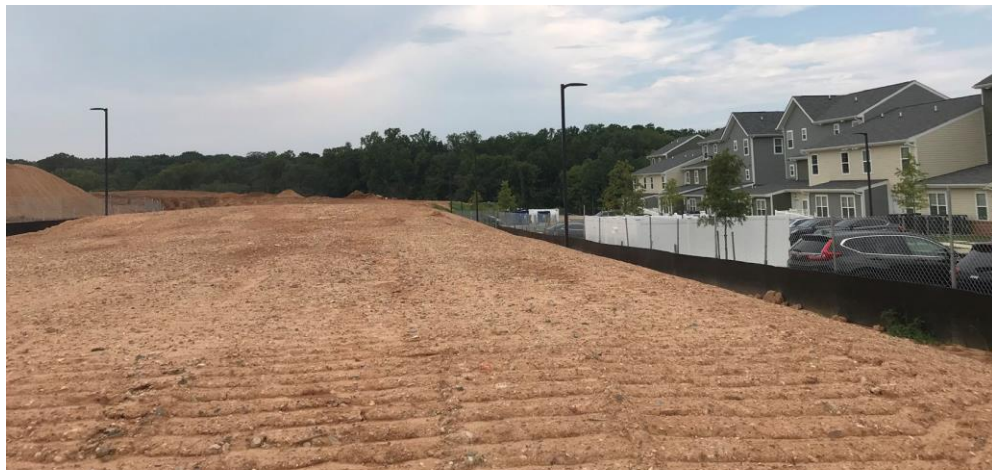
View facing west, Phase 3 lots in foreground, Phase 1 buildings to the right; RDA mass grading / site prep progress shown in foreground
